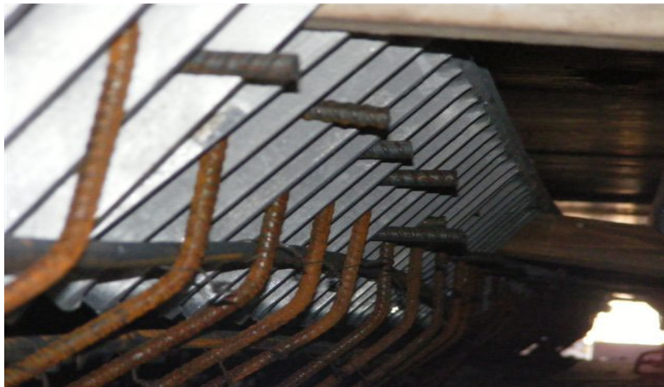
Fig. 16.12(B)-3 Photo of new Expansion device shown in Fig. 16.12(B)-2
