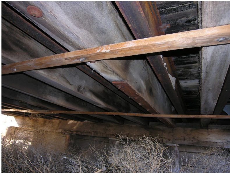
Fig. 16.12(H)-5 Photo of Added Steel Girder and Grader Blade on Timber Girder
